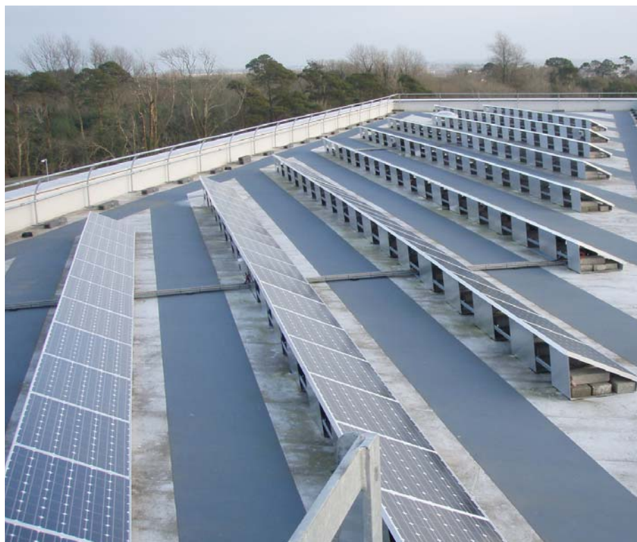
Figure 11: The EPA headquarters in Johnstown Castle, Wexford hosts the country's largest array of Photovoltaic (PV) solar panels in Ireland.
