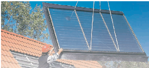
Figure 3.3. Solar energy from solar panels can complement other energy sources.
