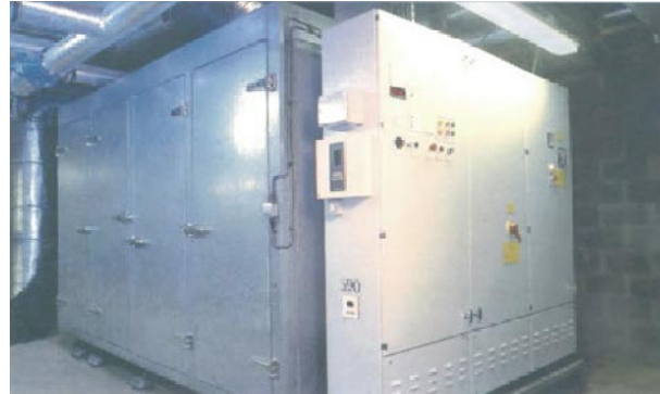
Figure A3.4. Typical CHP unit installed.
