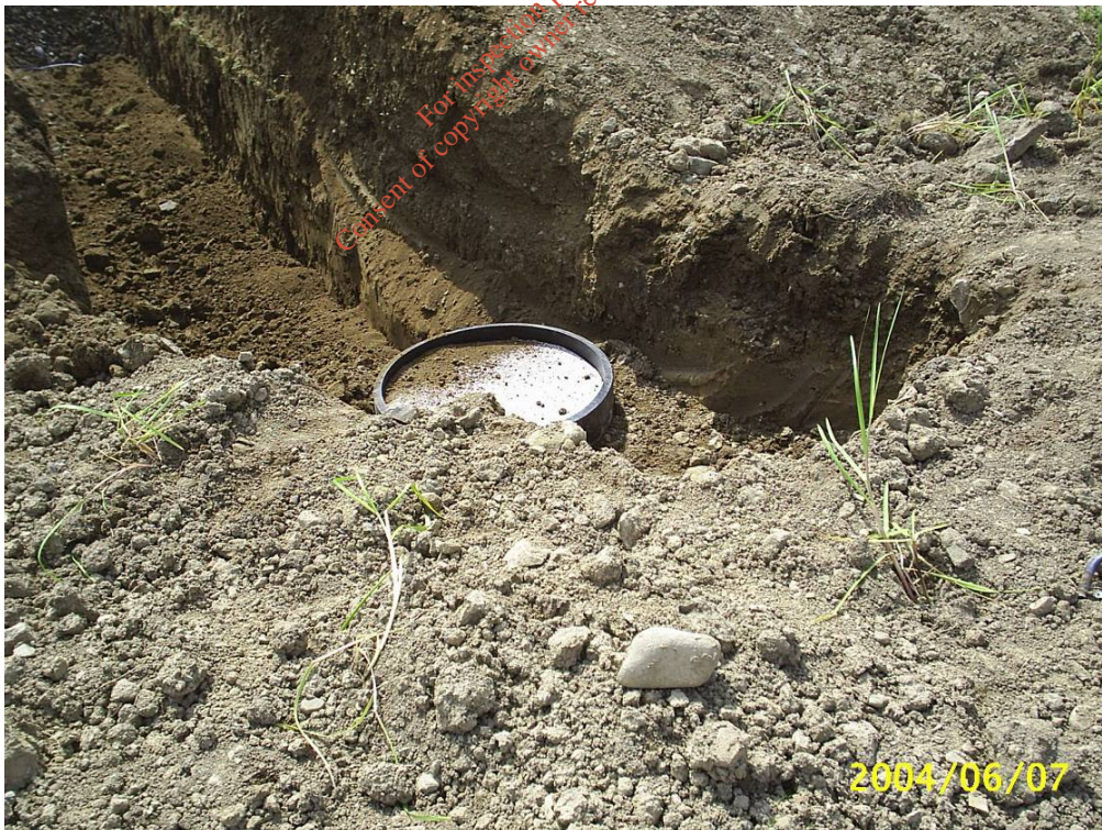
The above Lysimeter was installed 0.8m below the bottom of the wetland floor.
