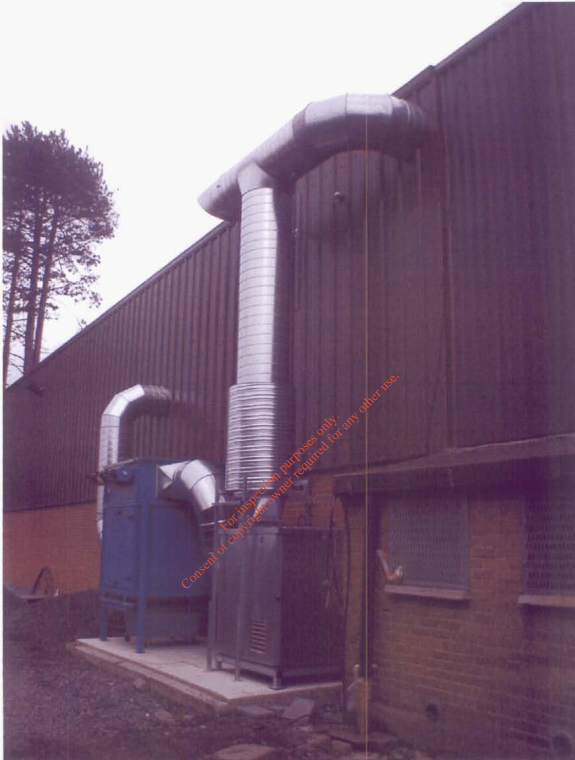
Figure 3: Dust Abatement Equipment for Welding Line
