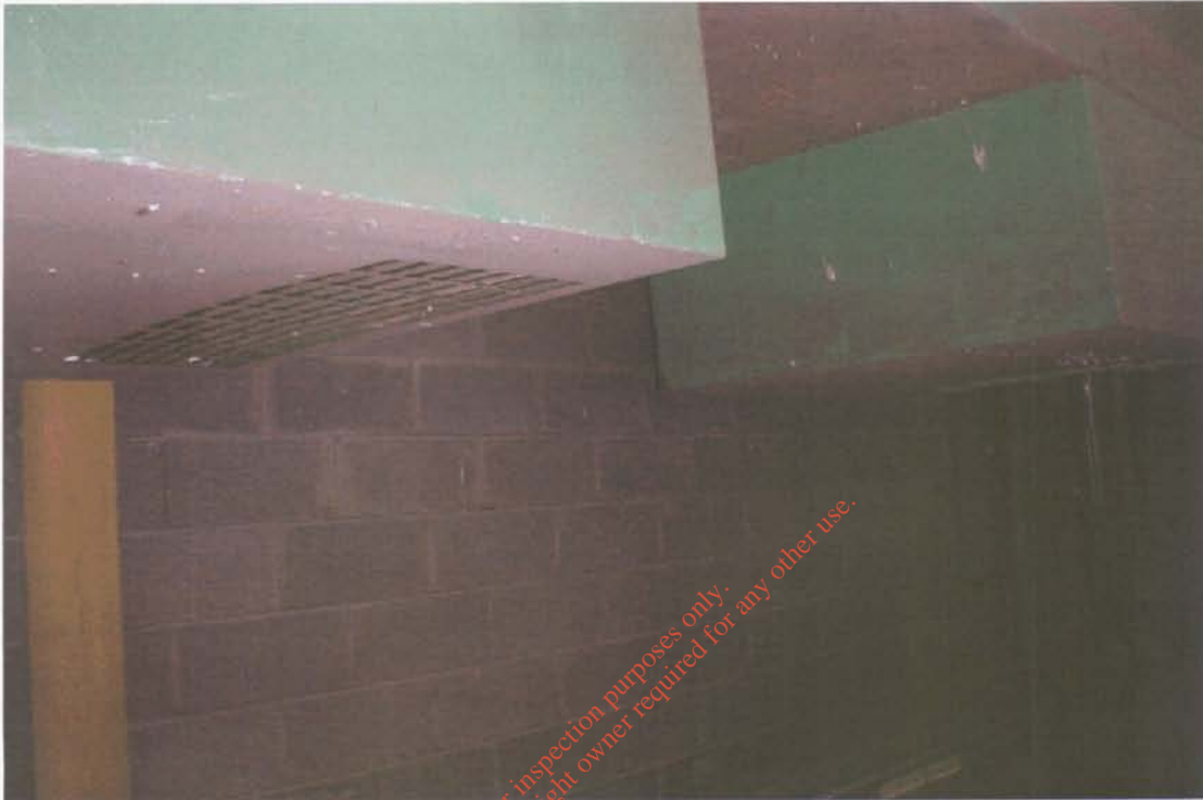
Figure 2: Vent details of Dust Abatement Equipment for Shot Blasting Line: D1 and D2
