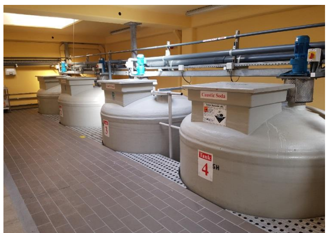
Photo 3 Caustic Soda tanks not in use and not banded
