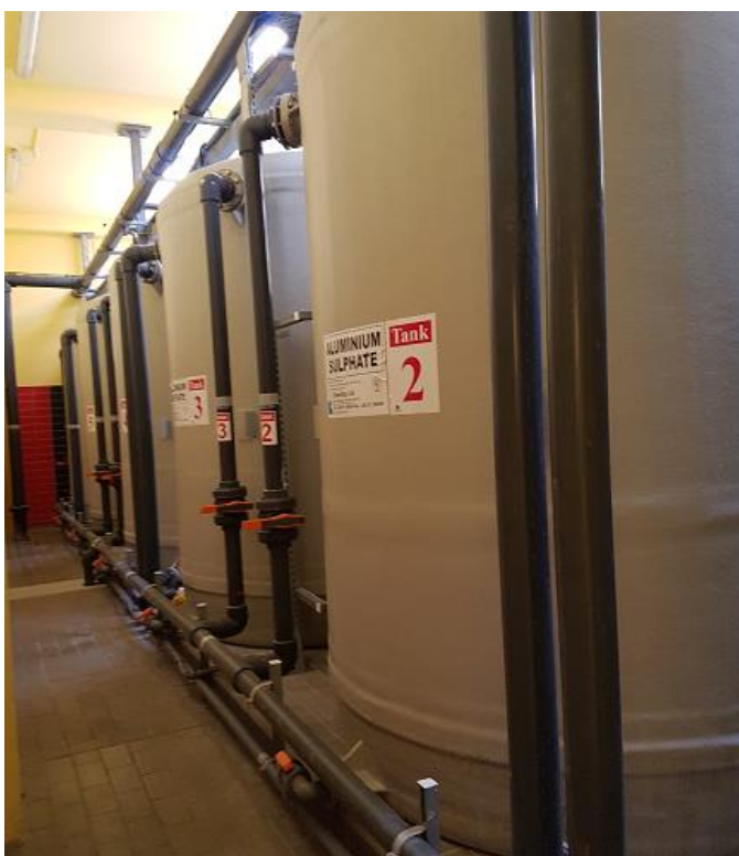
Photo 2 Alum tanks in use unbunded
