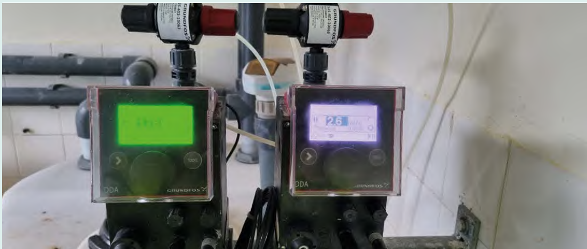
Main and backup chlorine (hypochlorite) dosing pumps assessed during an audit
