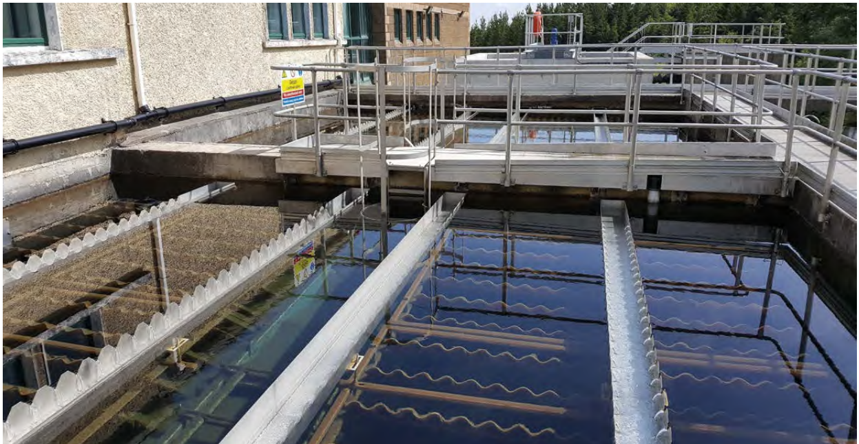
Figure 7: Water clarification tank – solids settle to the bottom and clarified water runs out in the channels
