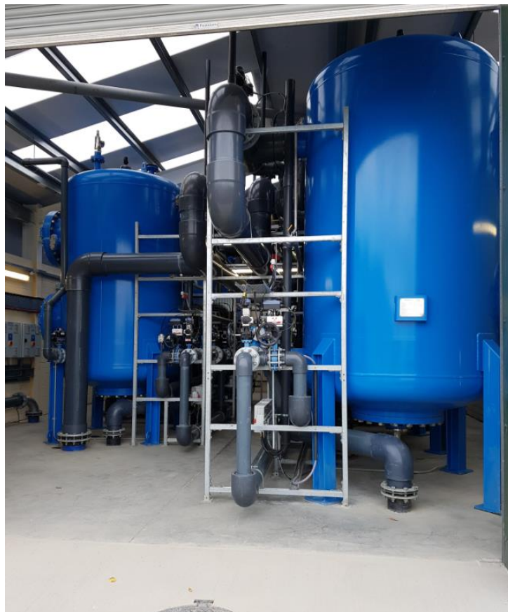
Photo 2 New Pressure Filters (Stage 1 on RHS & Stage 2 on LHS)
