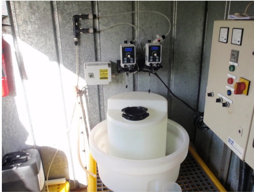
Photograph 1: Duty standby chlorine dosing pumps at the Ardtaggle reservoir, there was no chlorine residual monitor and no alarm.
