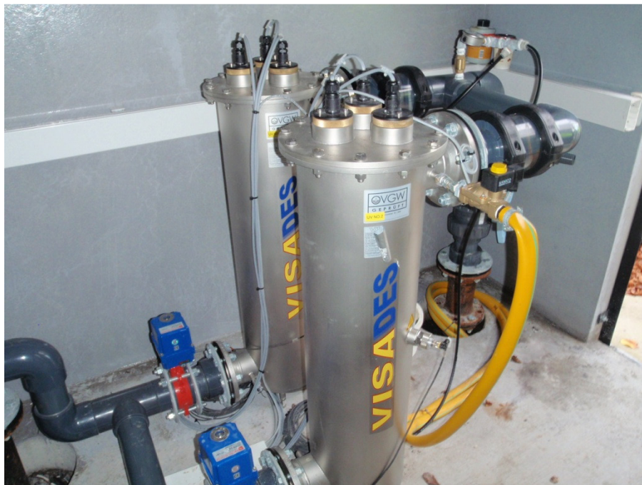
Photograph 2: Duty standby UV units at the O'Brien's Bridge supply. Two months UVI/UVT and flow data is required to ensure UV units have remained within their validation range at all times.
