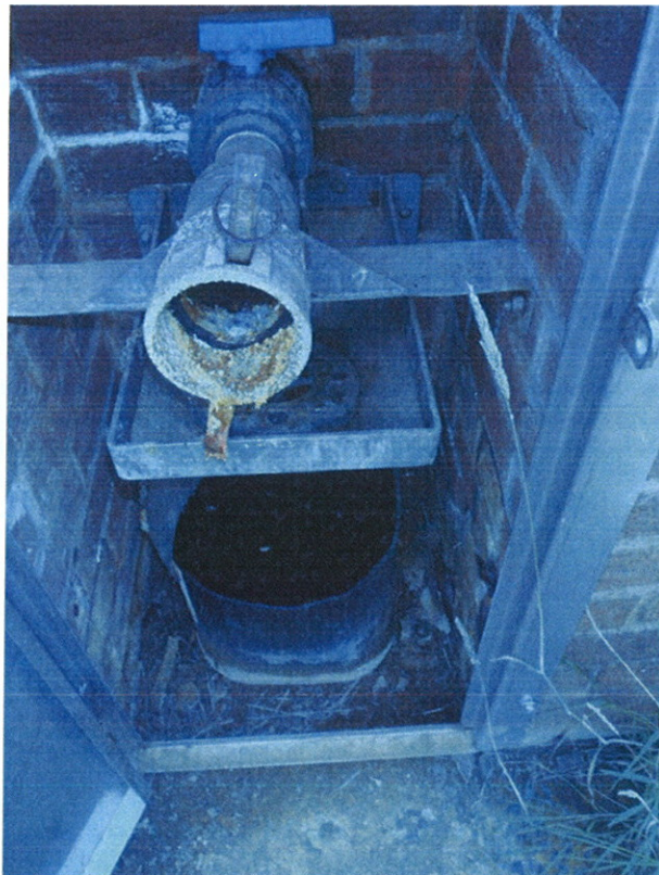
Photograph 6: Ferric delivery point; no cover or spill tray in place.
