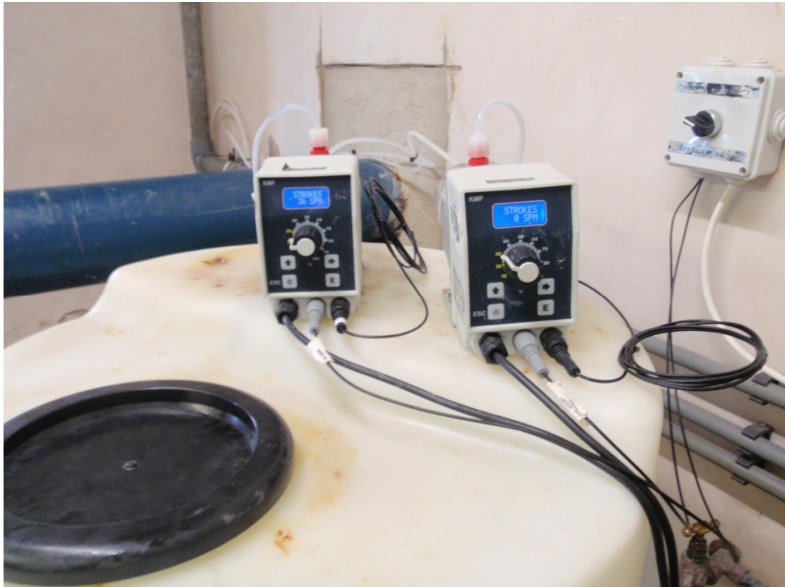
Photograph 1: Duty standby chlorine residual dosing pumps at the Flagmount water treatment plant. There is no auto switch over between the two pumps.
