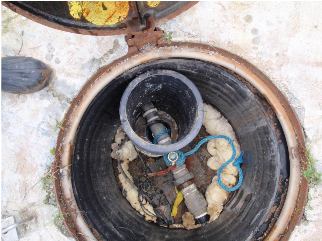
Photograph No. 1: Inadequate Wellhead Protection
