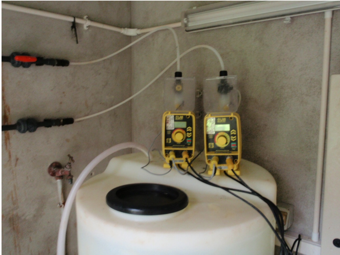
Photograph 1: Duty and standby chlorine dosing pumps at the Mountshannon water treatment plant. The chlorine residual monitor is located after the Mountshannon reservoir.
