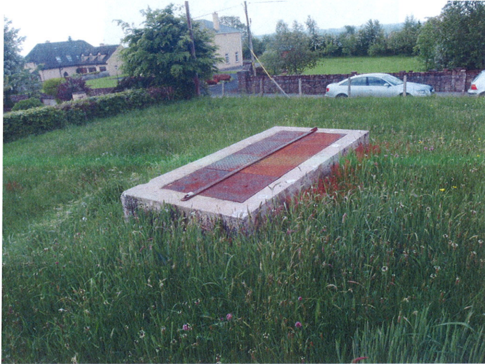
Photograph 6: The covers on the reservoir were observed not to be of the type that was sufficient to prevent surface water ingress. The reservoir was also observed to be covered in vegetation.
