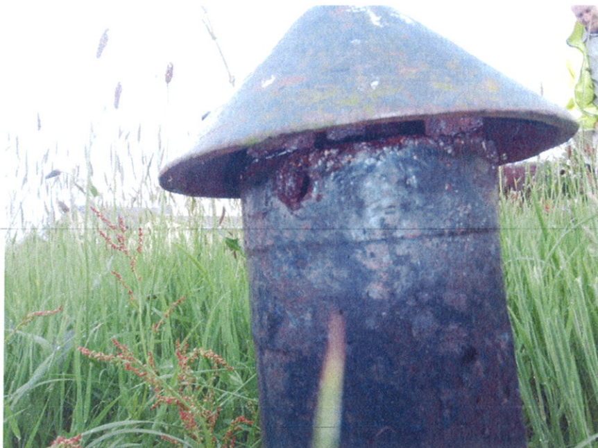
Photograph 5: Vents on reservoir were observed not to be secure against insects etc.
