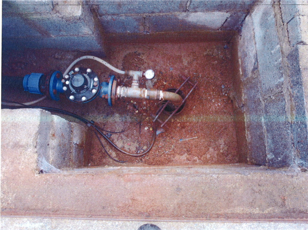
Photograph 2: Well head at Ardtaggle not constructed as per appropriate guidelines.
