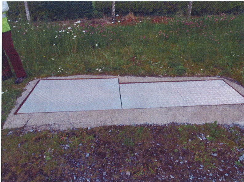
Photograph 3: The cover on the Ardtaggle reservoir was also observed not be effective against surface water ingress.
