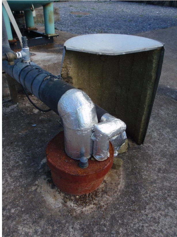
Photograph 1: Rusting cap on borehole.
