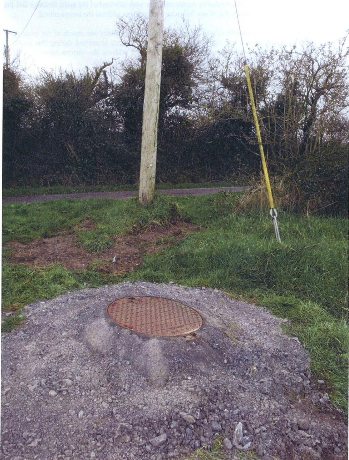
Photograph 1 – Borehole locality. Note no formal drain at road verge and potential for surface water drainage in the direction of the well head.
