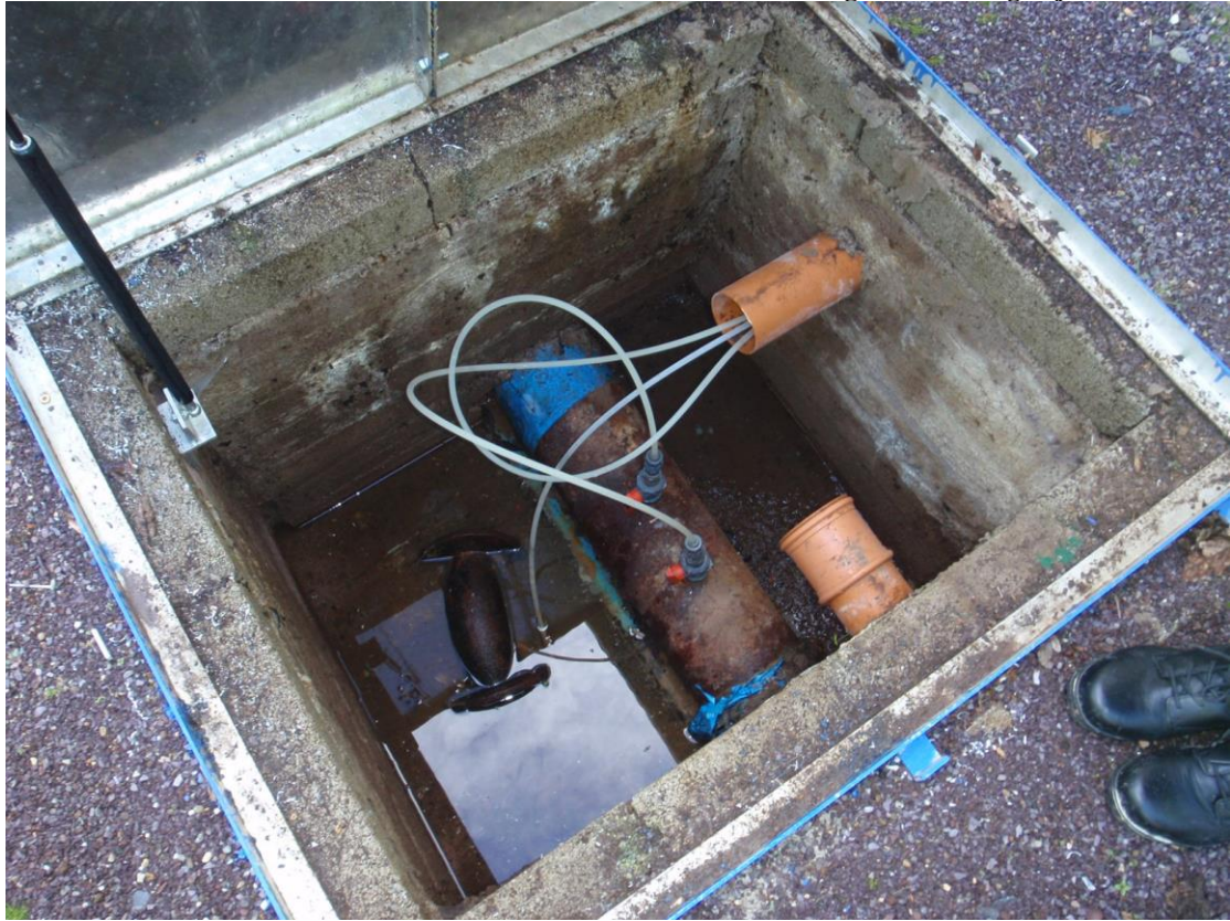
Photo No. 1 – Visible Water on Floor of Manhole Chamber Housing PAC Dosing Injection Points
