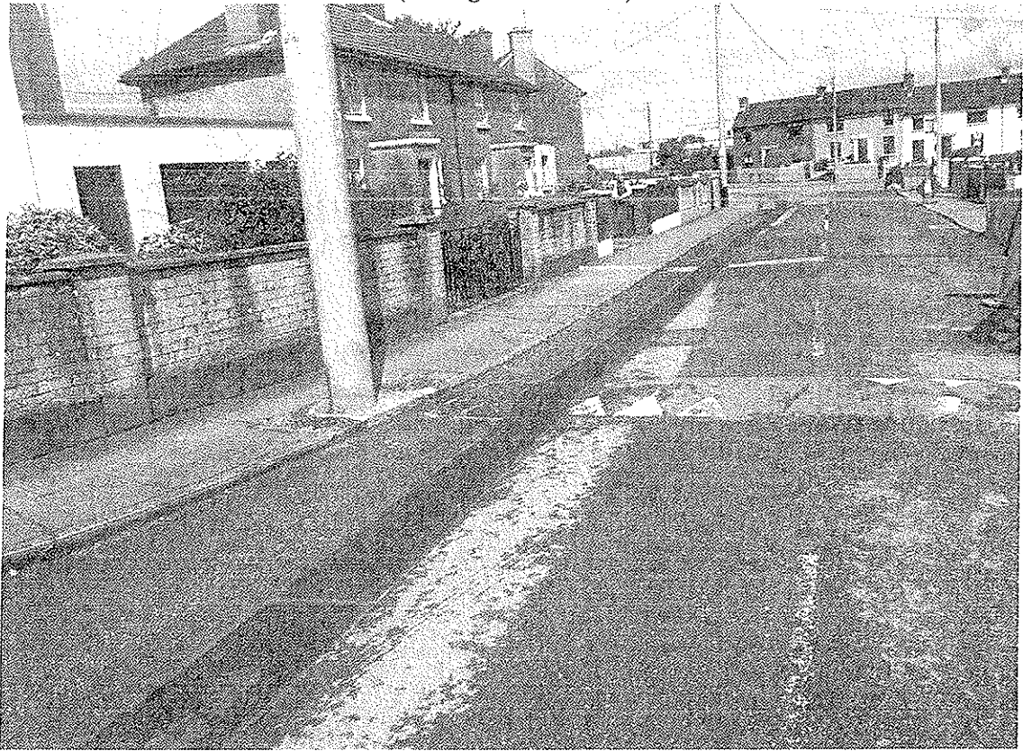
Photograph 3: Evidence on street surface of work completed to install new main at Glenanaar Row (looking East and West)
