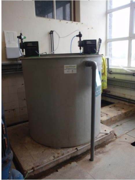
Photograph No. 1: PAC day-tank not banded.
