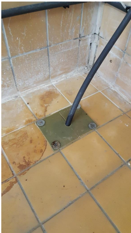
Photograph No. 2: Hole Above Clear Water Sump
