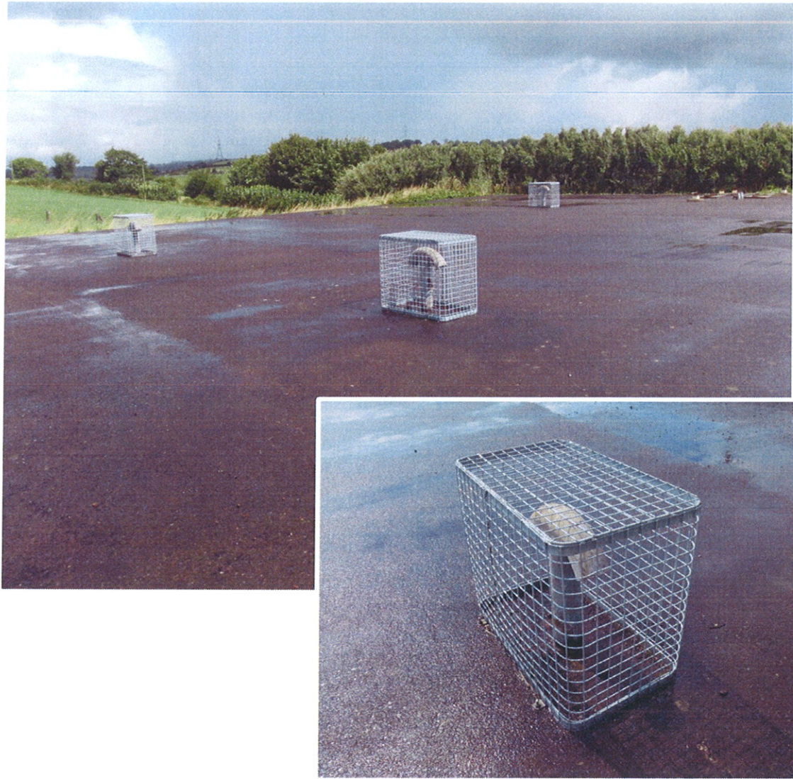
Photograph No. 3: Reservoir vents – secure against vandalism but no mesh in place.
