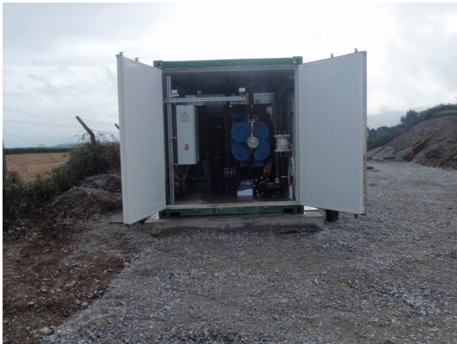
Photograph 1: One of the micro filtration unit, still under commission.
