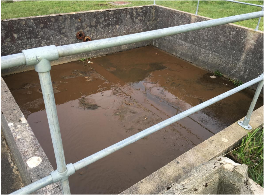
Photo 1 Holding tank for expended backwash water and sludge bleeds
