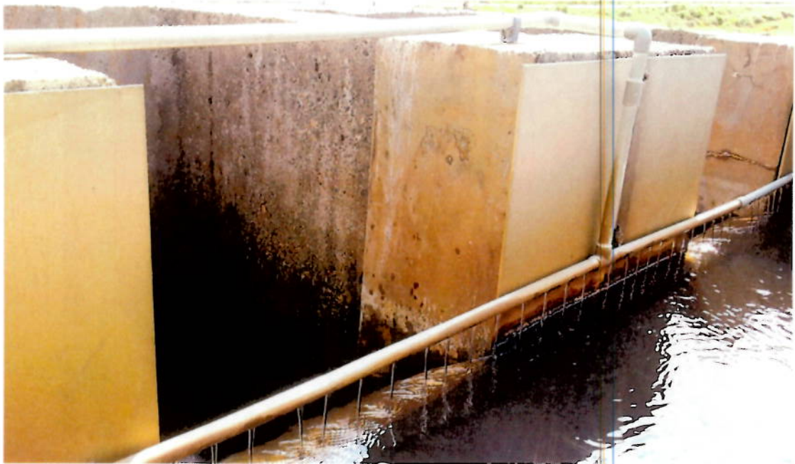
Photo 4 Poly being dosed in contact tank prior to clarifiers
