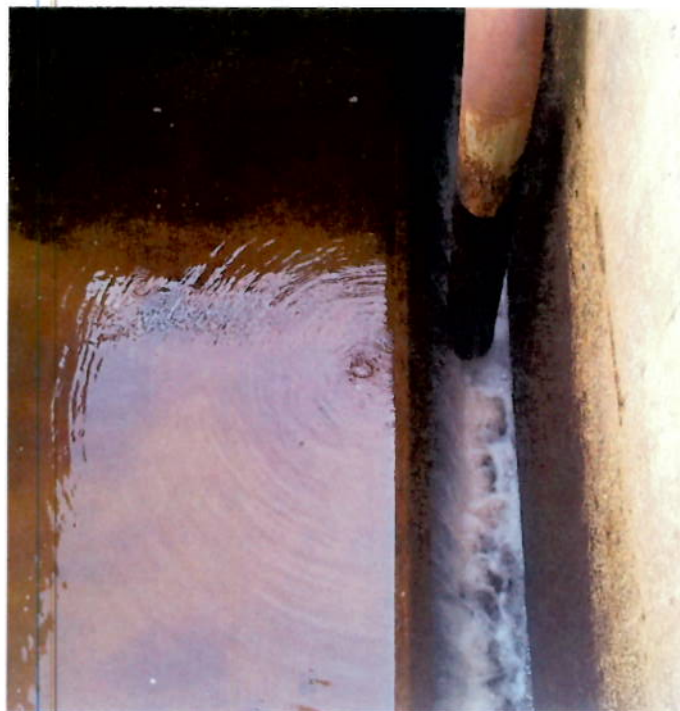
Photo 7 Air valve not fully closed giving rise to air bubbles during the wash water stage at backwash of Filter No. 3.
