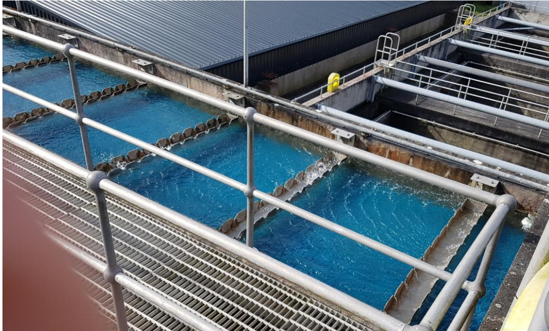
Photo 5 Strong winds producing surface water currents in the clarifier and affecting settled water entering decanting troughs
