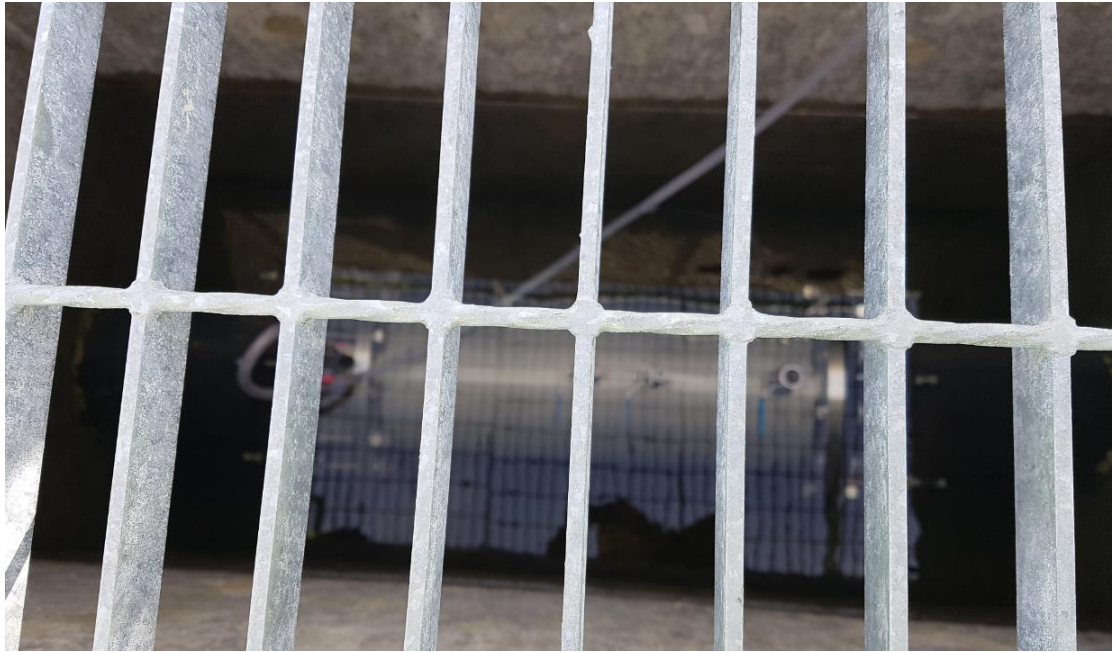
Photo 3 Rainwater has collected in the aluminium dosing point chamber and submerges the transfer pipe
