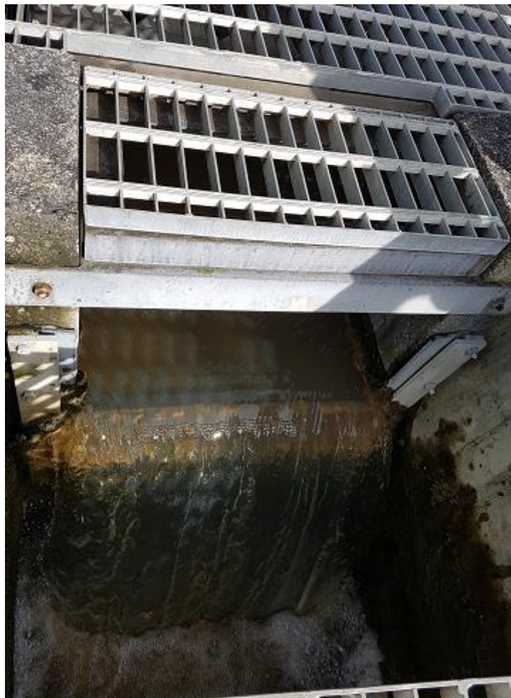
Photo 4 Weir post poly dose prior to entry to clarifiers
