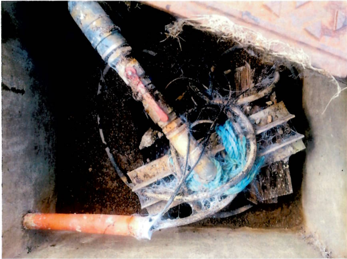
Photo 1. Borehole of the Cineal Feicin PWS (note no cover on borehole).
