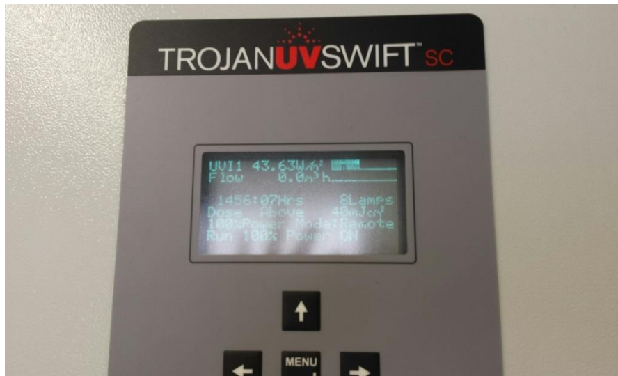
Photo 2: UV Reactor No. 1 control panel showing 0.0 m 3 /hr flow during operation
