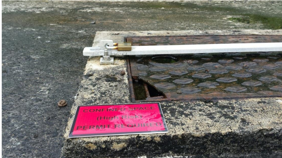
Photo 1: Damaged manhole cover at Kilcarna rainwater spring source (note the bird droppings in the immediate vicinity present a risk of contamination of the raw water source)
