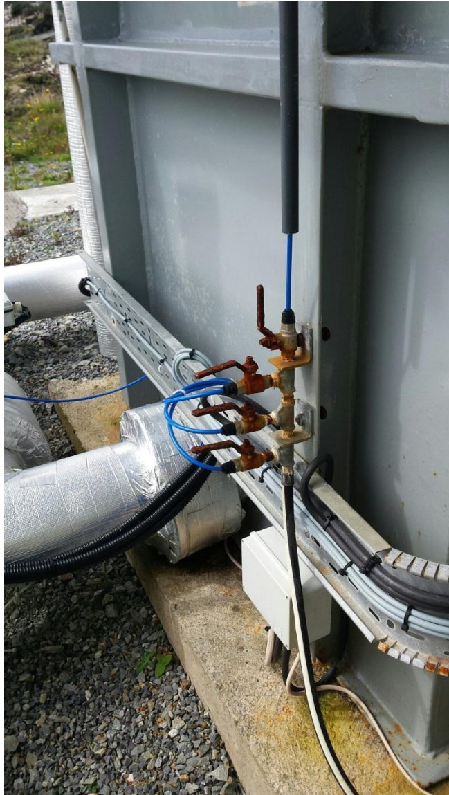
Photo 1: Corrosion of chemical injection points into the DAFF unit
