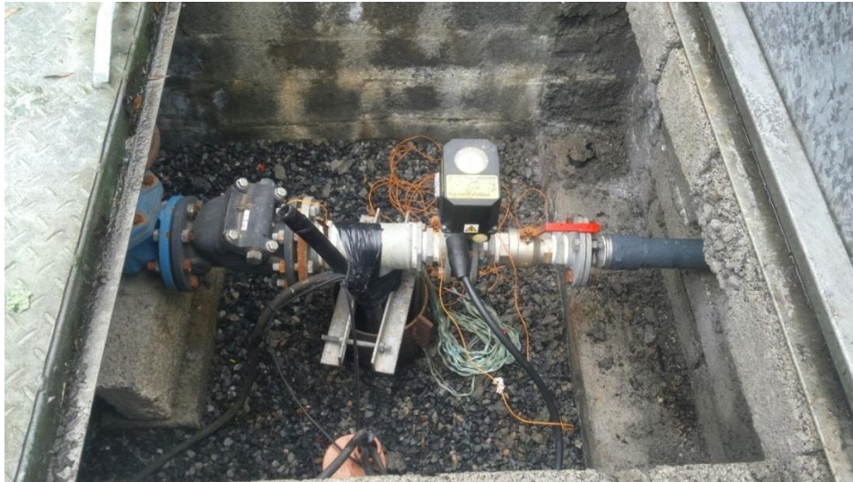
Photo 1: Uncapped borehole at Kilconnell water treatment plant
