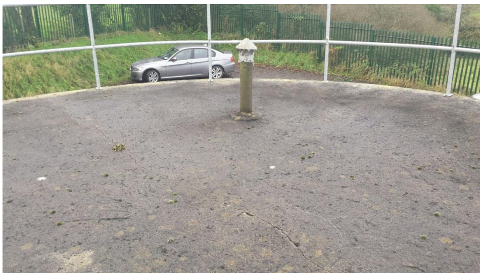
Photo 3: Cracks on roof of Kilconnell reservoir.
