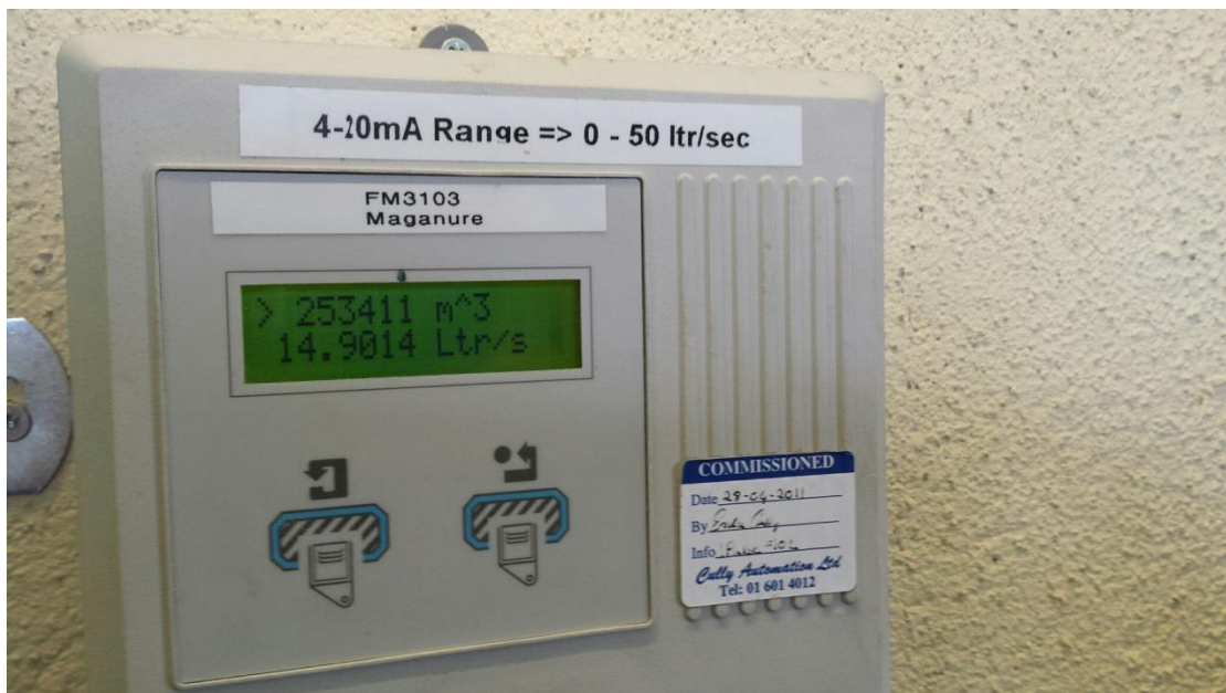
Photo 2: Flow meter label - no record of calibration/service since it was commissioned in 2011
