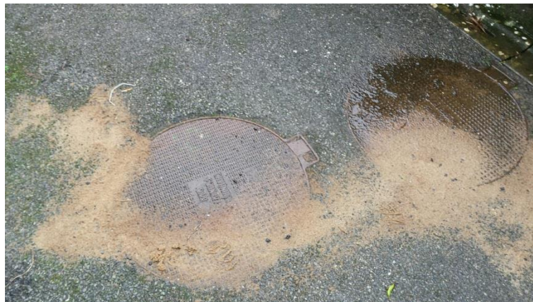
Photo 2: Sand on the ground beside the filter backwash pipework/manholes at Lake Road WTP
