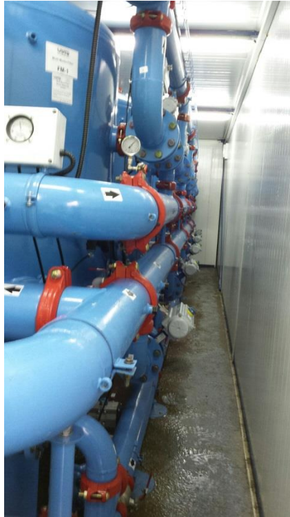
Photo 1: Sand on the floor in the pressure filter room at Lake Road WTP
