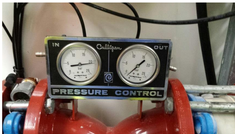
Photo 3: Broken outlet pressure gauge on Culligan Filter No. 2 at Knockanima WTP.
