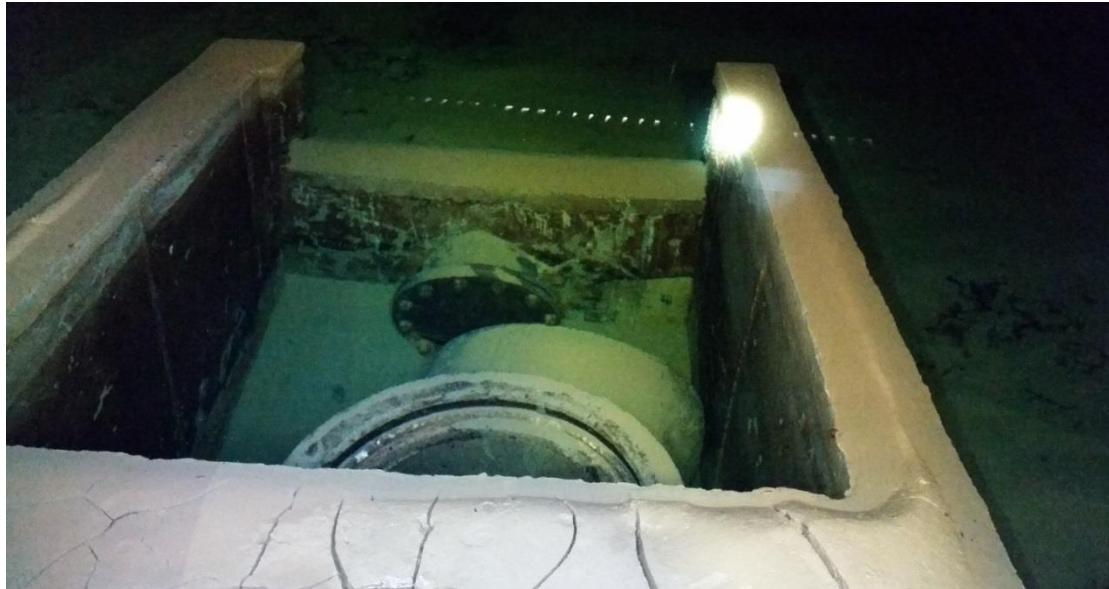
Photo 1 Spring source covered - note thin layer of fine silt on inlet
