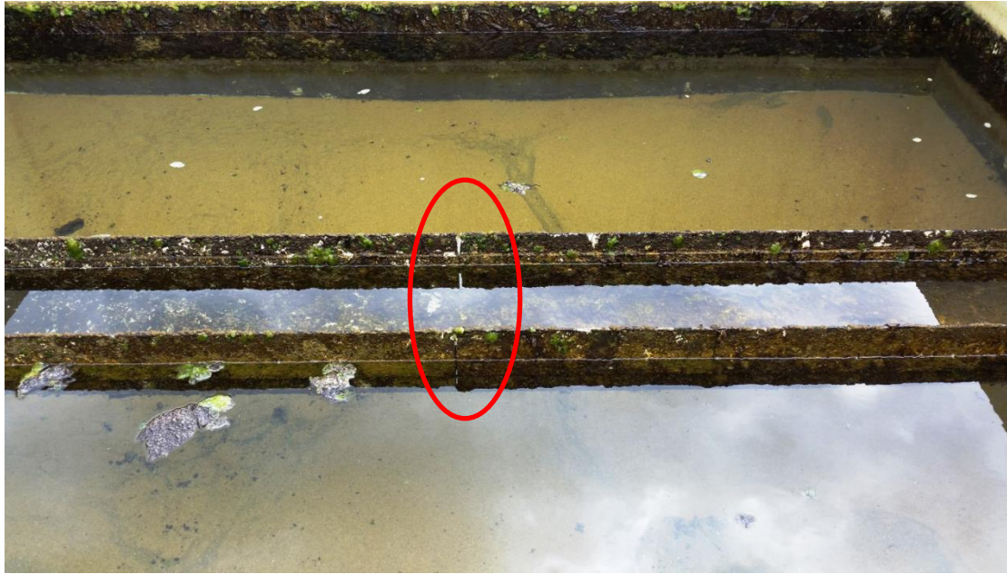
Photo 3 Filter No. 1 showing algae on filter walls and channel and gap in channel (circled in red)
