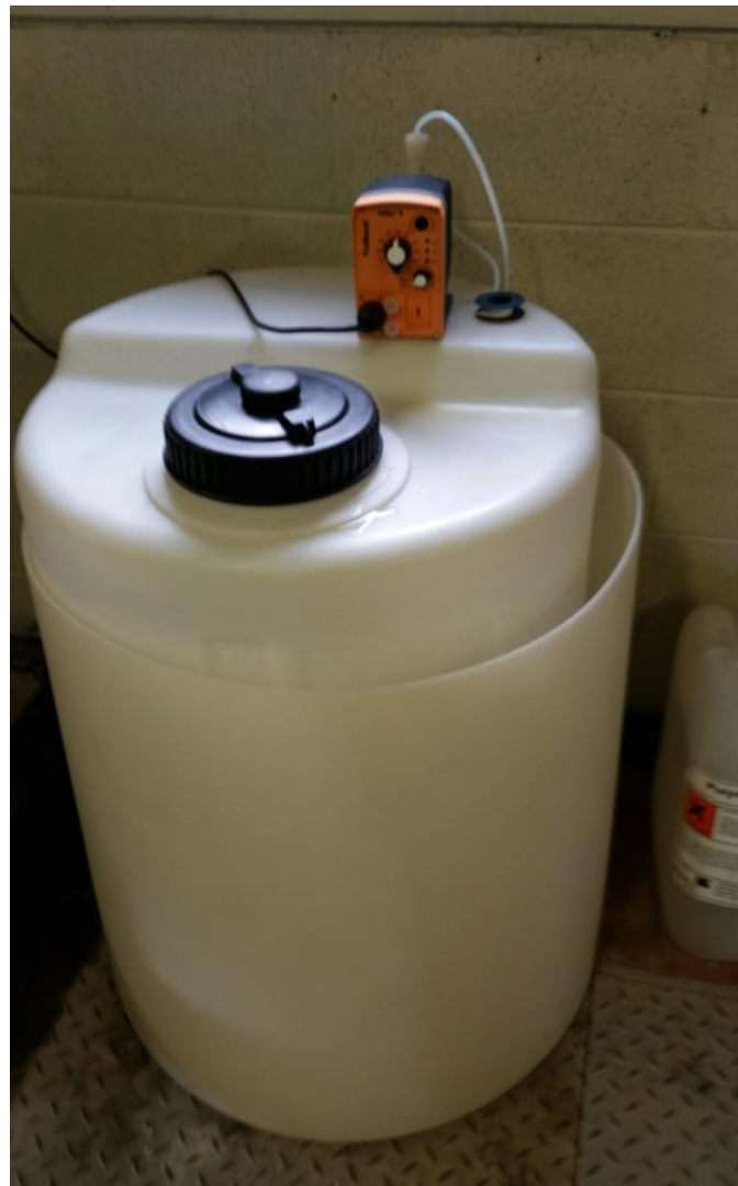
Photo 2 Liquid Poly Aluminium Chloride (PAC) dosed intermittently pre-filtration
