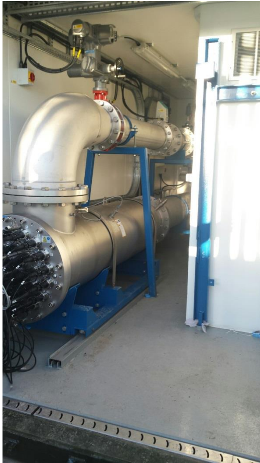
Photo 1: Containerised UV disinfection system at Williamstown WTP
