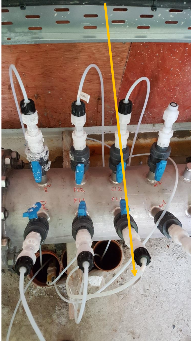
Photograph 1: Sodium hypochlorite dosing line - vulnerable to accidental damage.
