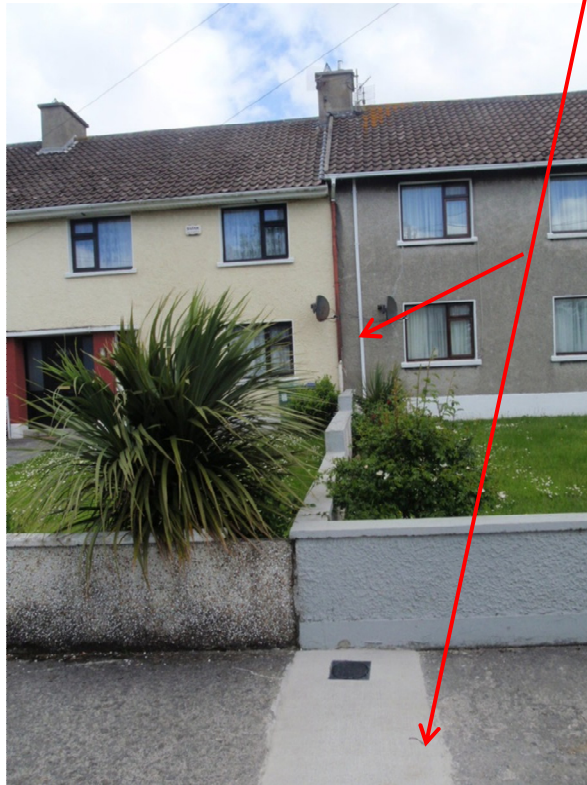
Photograph 7: St Brendan's Park. Trench Scar and external plumbing.
