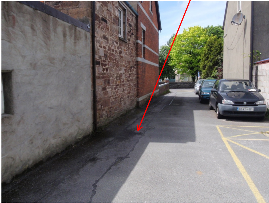
Photograph 2. Cloonmore Road, trench scar in alley way.
