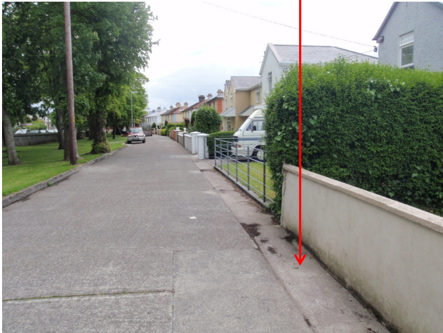
Photograph 5: Cloonbeg Terrace, trench scar observed at stopcocks.
