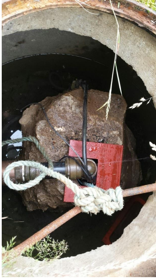
Photograph No. 2: Poor wellhead protection and standing water in the borehole chamber
