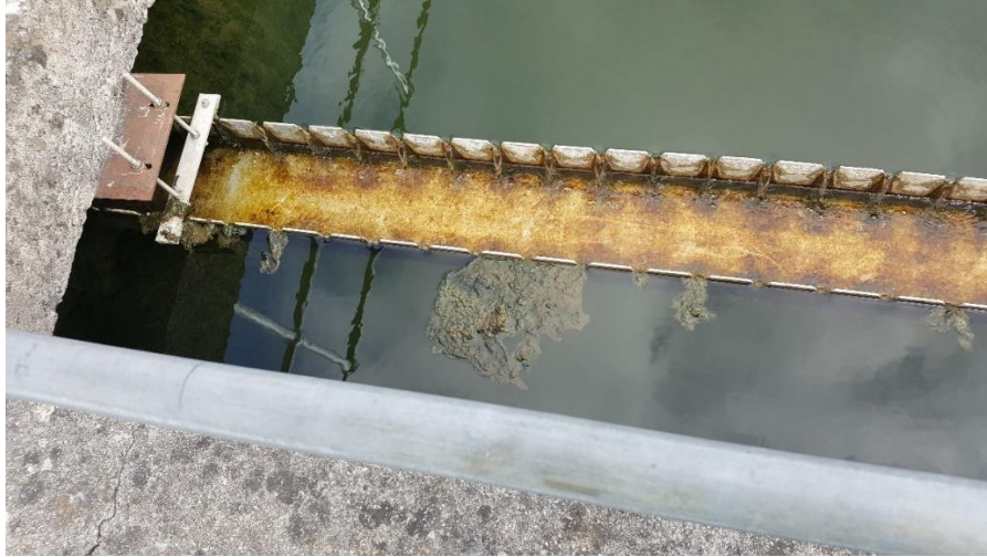
Photo 1: Flocs/algae collecting in decanting channel of clarifier
