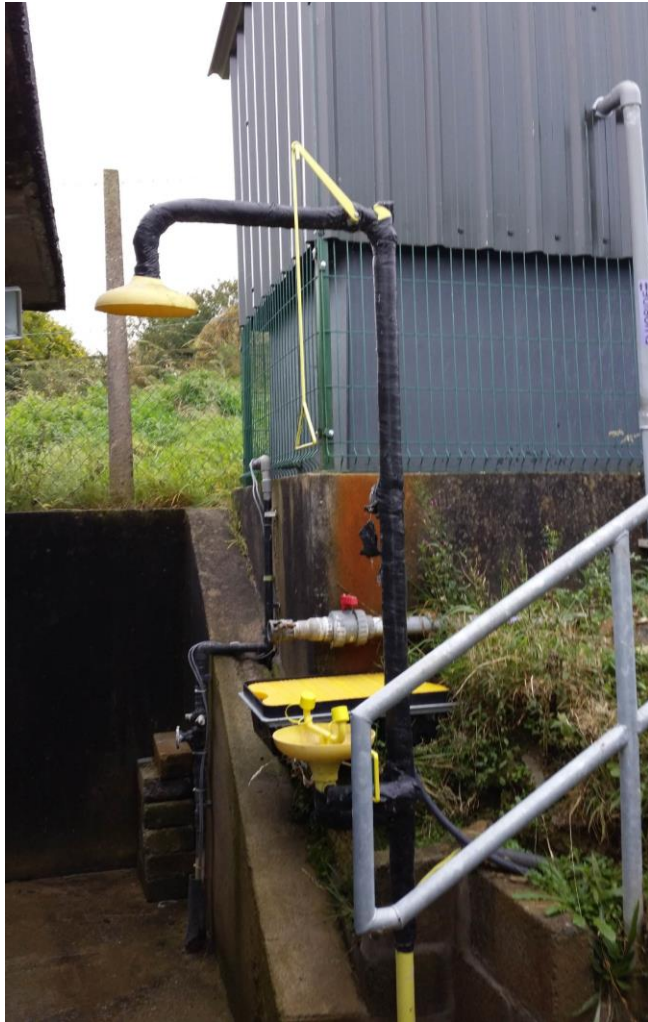
Photograph 1: Unbunded hydrofluorosilicic acid fill point
