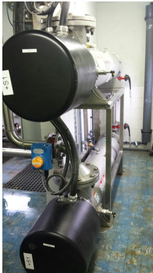
Photo 2: New duty and standby UV disinfection units
