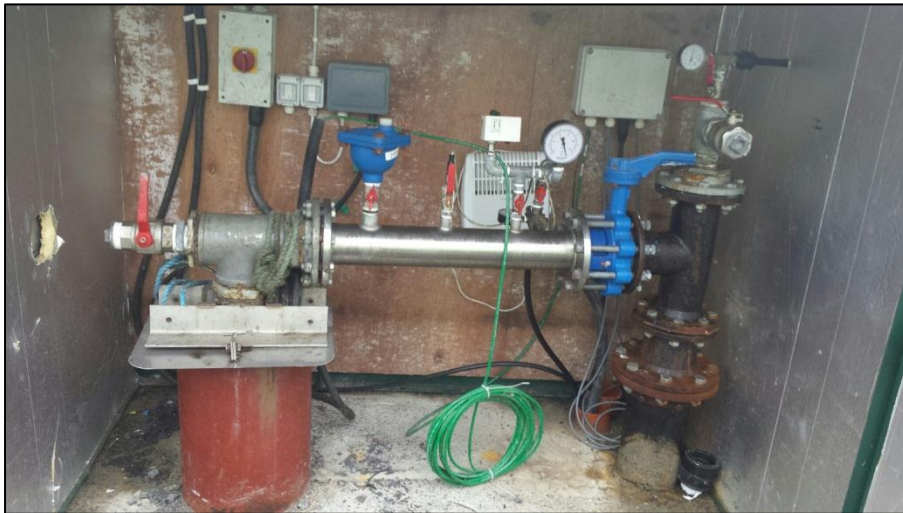
Photo 3: Borehole cover at Eyne No. 1
