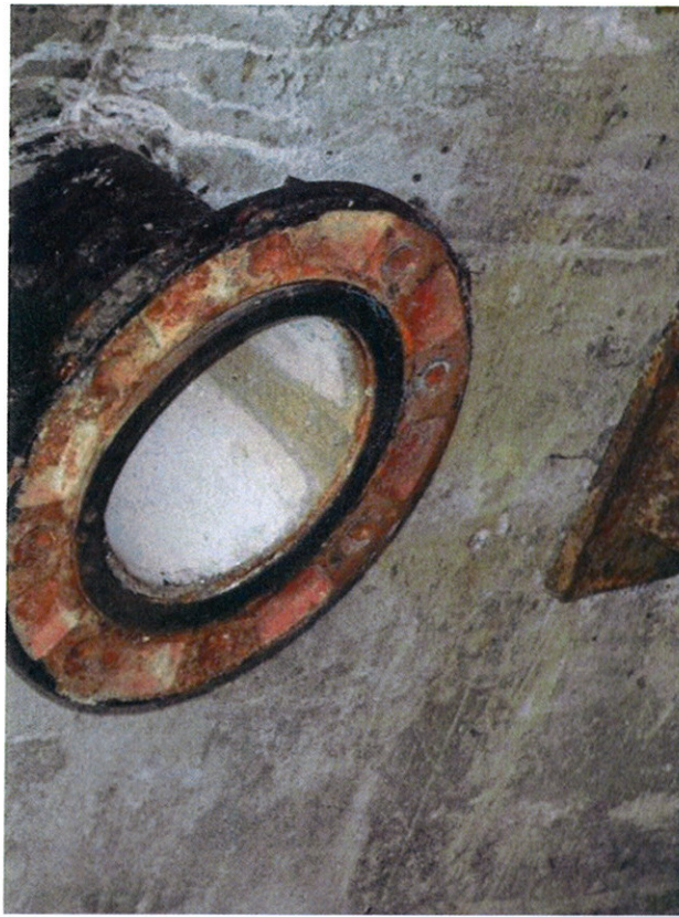
Photograph 3: Overflow pipe in wellhead chamber, Borehole 1, Derrygarran
