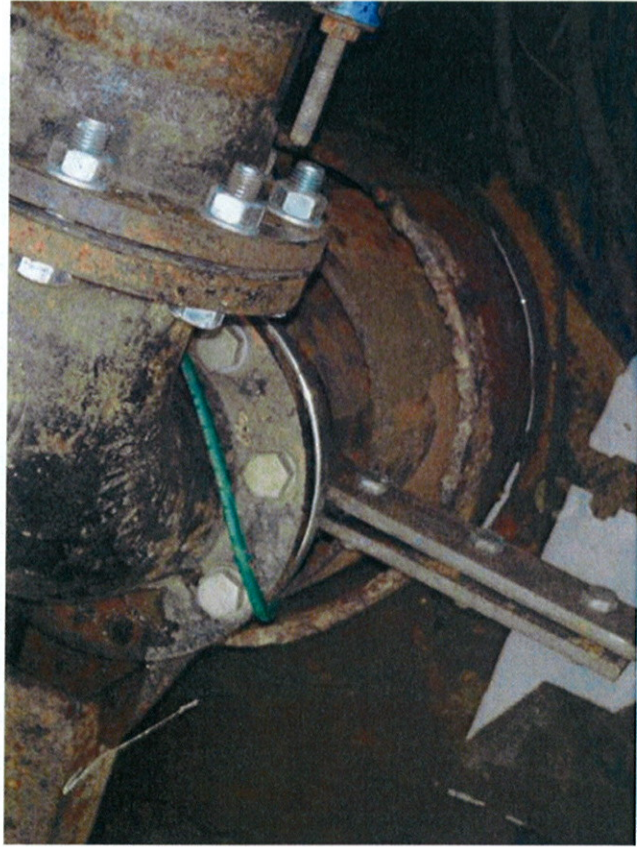
Photograph 2: Unsealed wellhead, Borehole 2, Derrygarran
