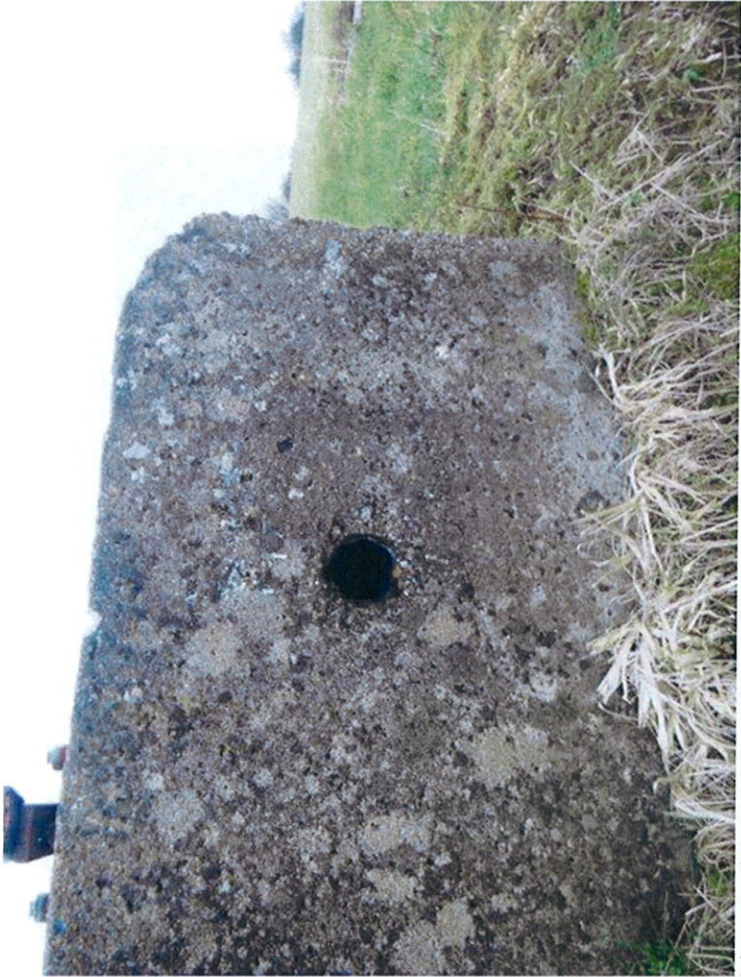
Photograph 5: Pipe from access hatch on reservoir 1 at Kilminchy plant
