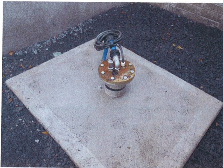
Photograph 1: Well head. Kiosk to be placed over well head.
