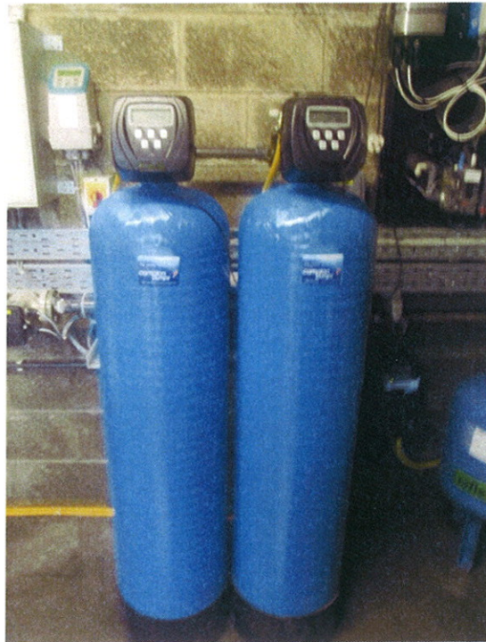
Photograph 2: Manganese and iron filters.
