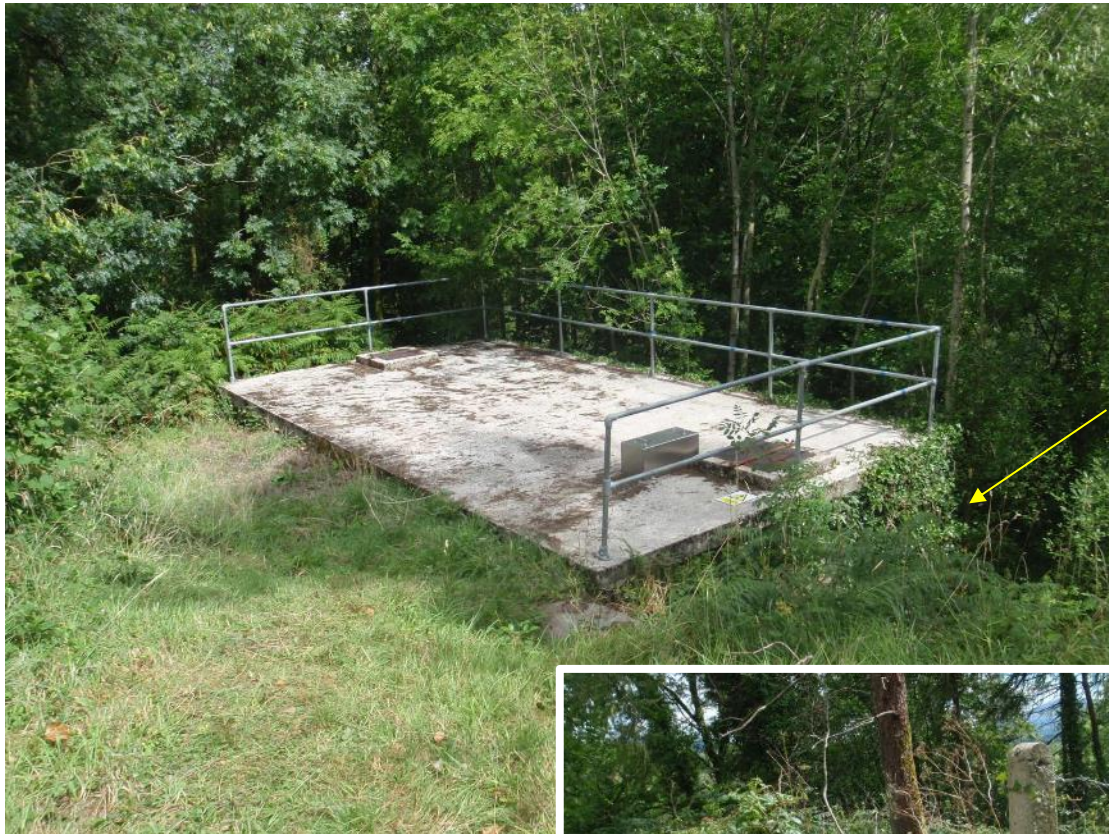
Photograph 2: Reservoir: ivy on side of structure and perimeter fence not stock proof.
