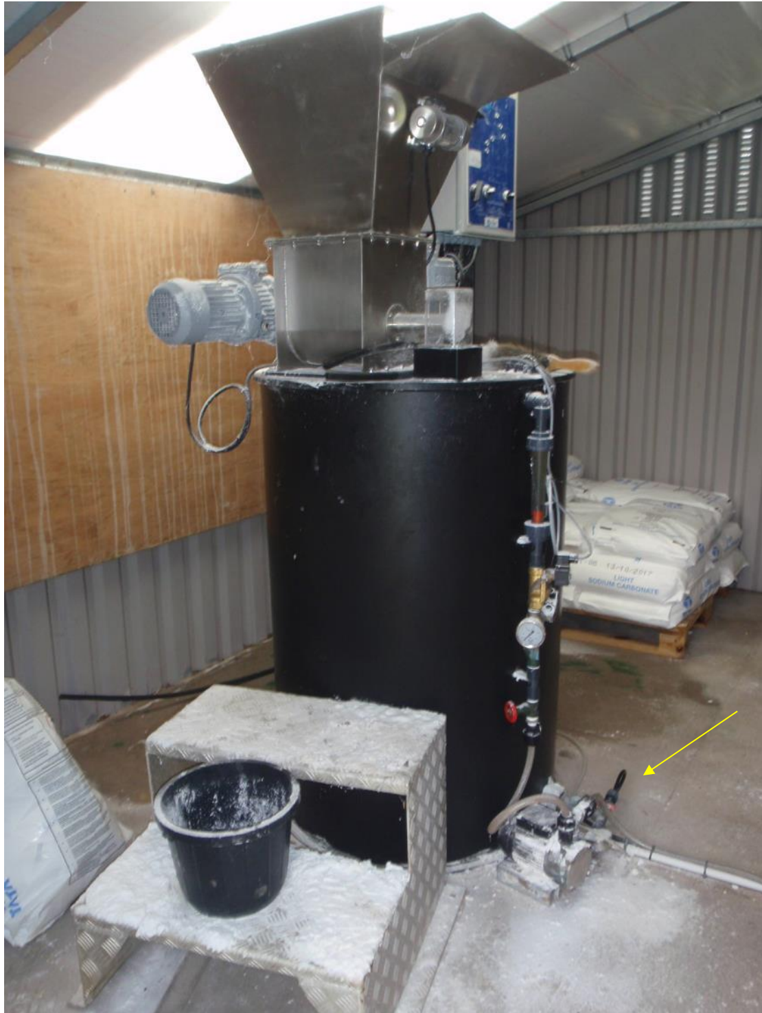
Photograph 1: Soda ash dosing pipework – potentially vulnerable to damage.
