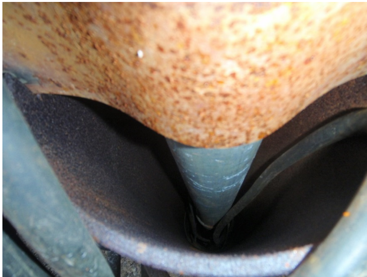
Photograph 1: No grouting between the inner and outer casings of the bored well.
