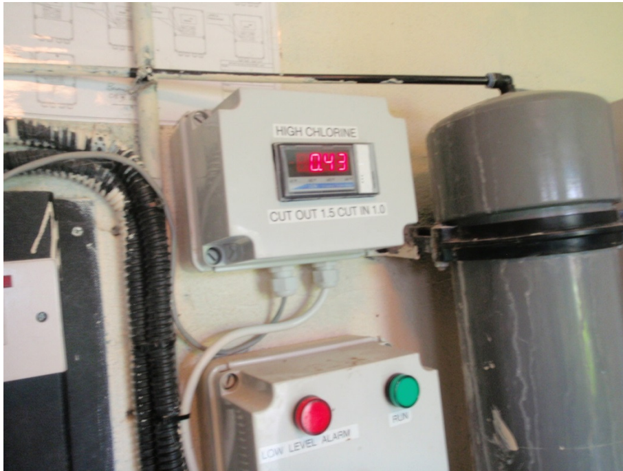
Photograph 3: Reading on chlorine monitor 0.43mg/l, reading on hand held chlorine monitor was 0.62 mg/l.
