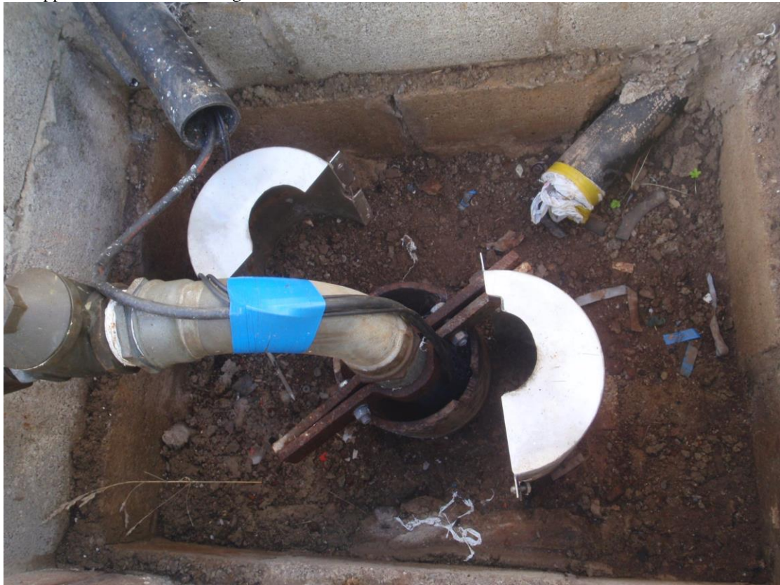
Photograph No. 1: Keating's Well (with cap removed for inspection). Inadequately sealed well head and apparent insufficient casing of the borehole shaft.
