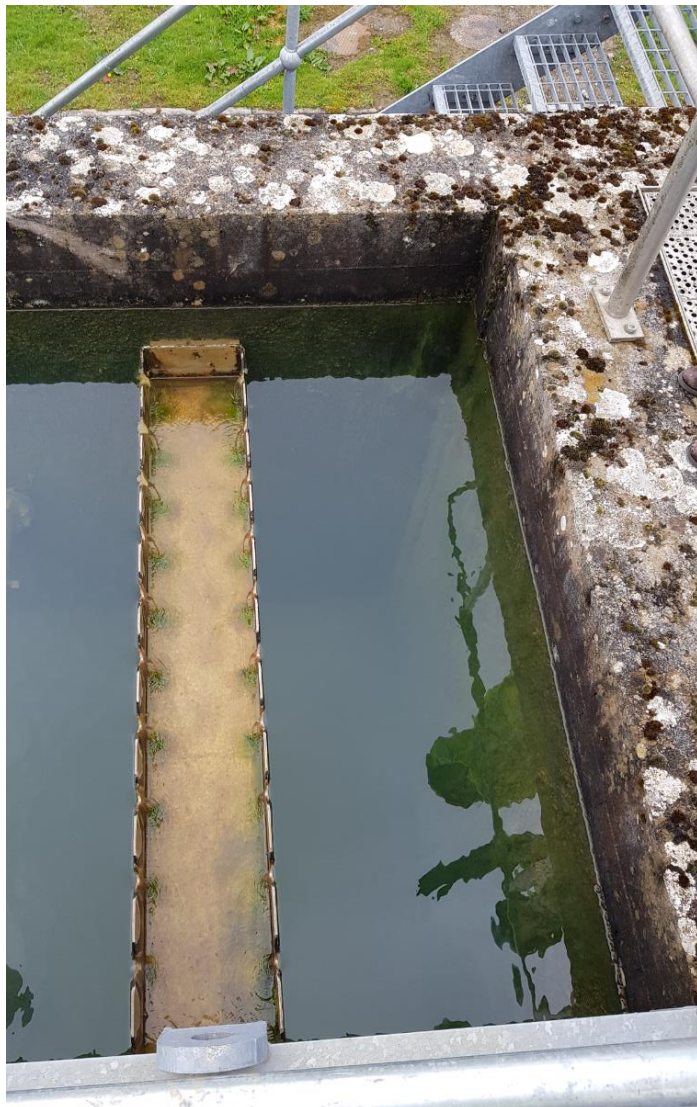
Photo 3 Algae on decanting channels and walls of clarifier
