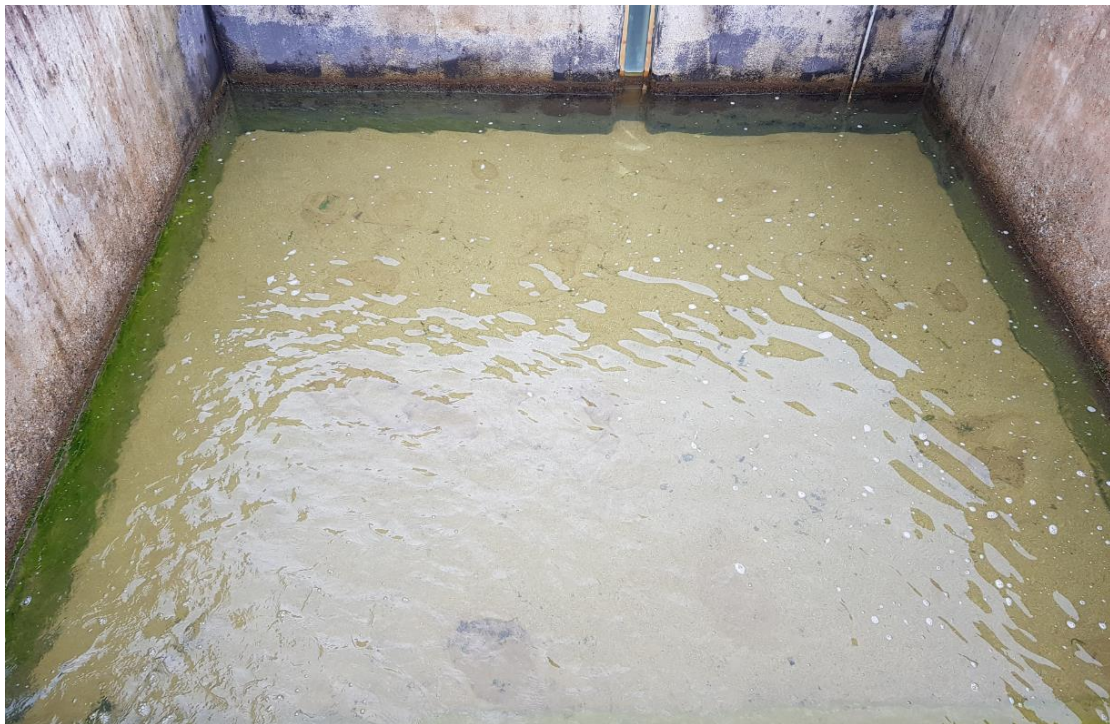
Photo 5 Traces of boils on Filter Media
