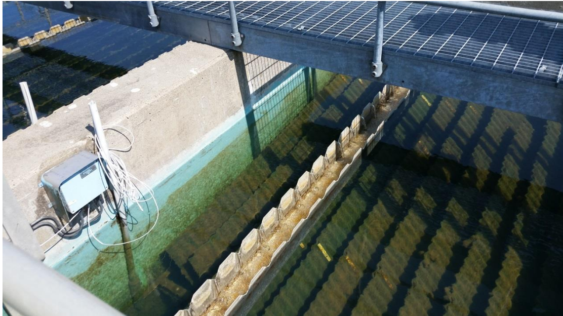
Photograph 1: Floc on walls of clarifier 2
