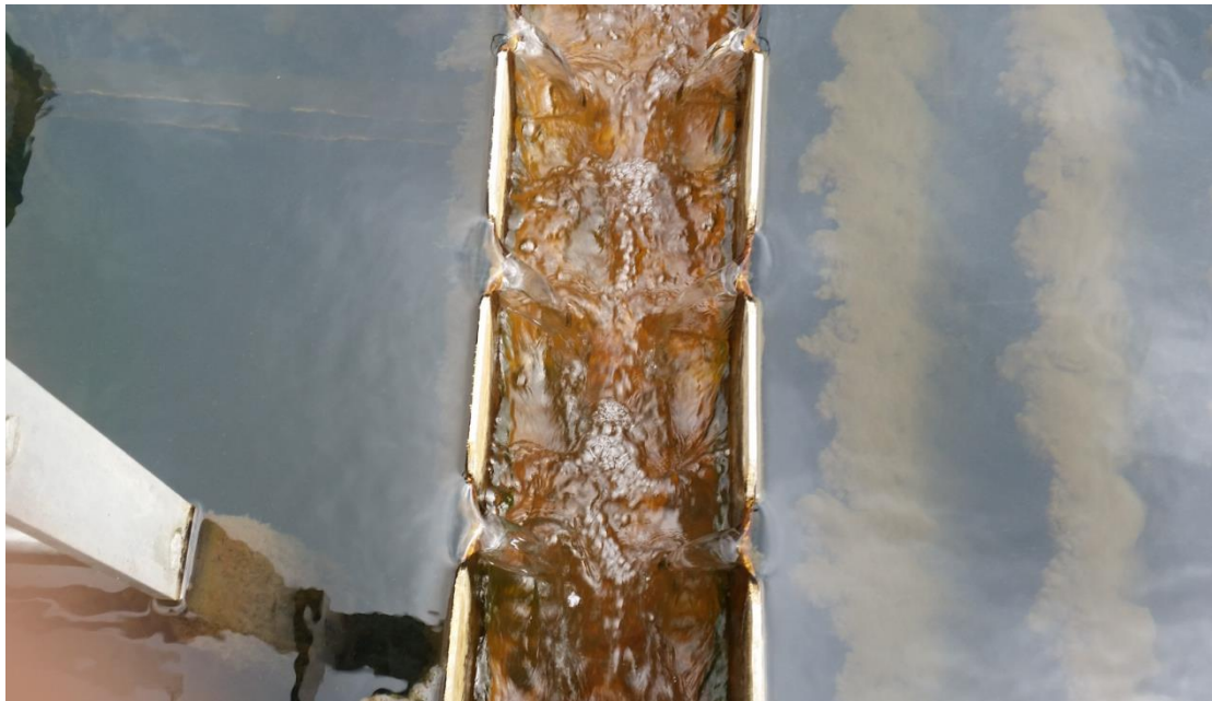
Photo 1 Pin floc and sludge build up on clarifier
