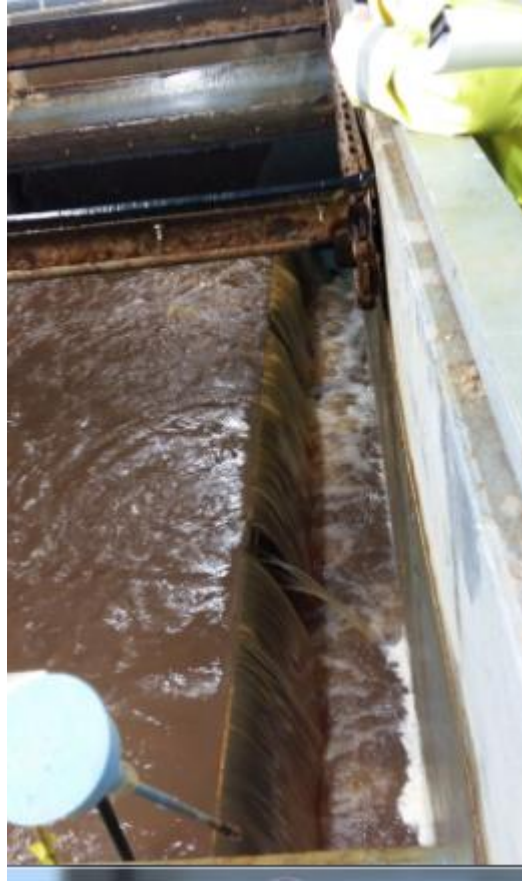
Photo 3 Backwash on DAFF Unit No 1 – water escapes via gap in weir
