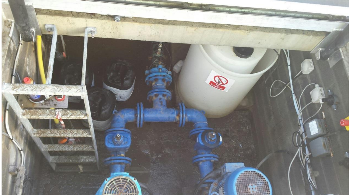
Photograph 2: View into combined chlorine booster and pump station underground chamber.
